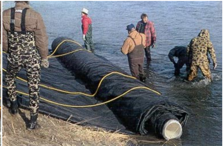
2. Ropes extend to circle under AquaDam and back to anchor pipe. On bank the AquaDam begins filling.
